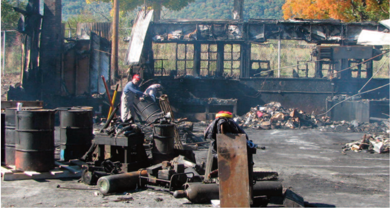
Remains of the Sequatchie County Highway Department office and shop after a devastating fire.
